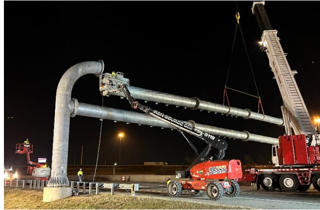
Double mast steel monopipe overhead structure.
